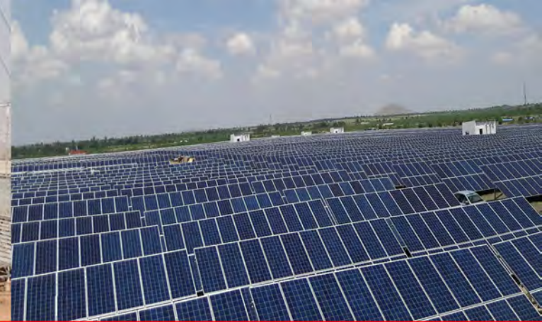
Solar PV Plant with Seasonal Tilt in Karnataka
