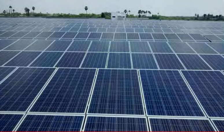
Solar PV Plant with Seasonal Tilt in Tamil Nadu
