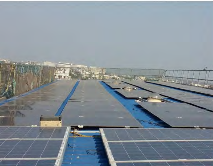
Grid Paralleled Rooftop Solar PV Power Generation System installed in our Office Premises
